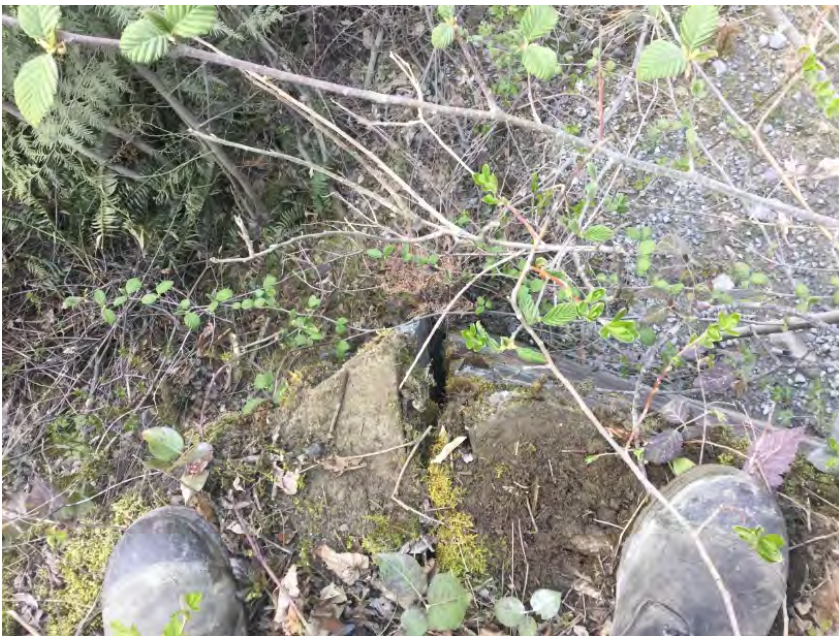
Downstream left bank precast wingwall - slight out of alignment with ballast wall
