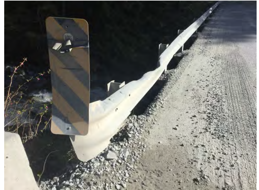
Guardrail damage upstream right bank
