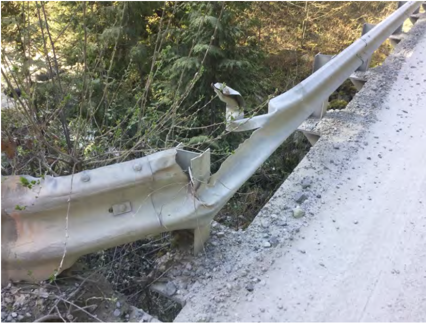
Damage noted to downstream left bank guardrail
