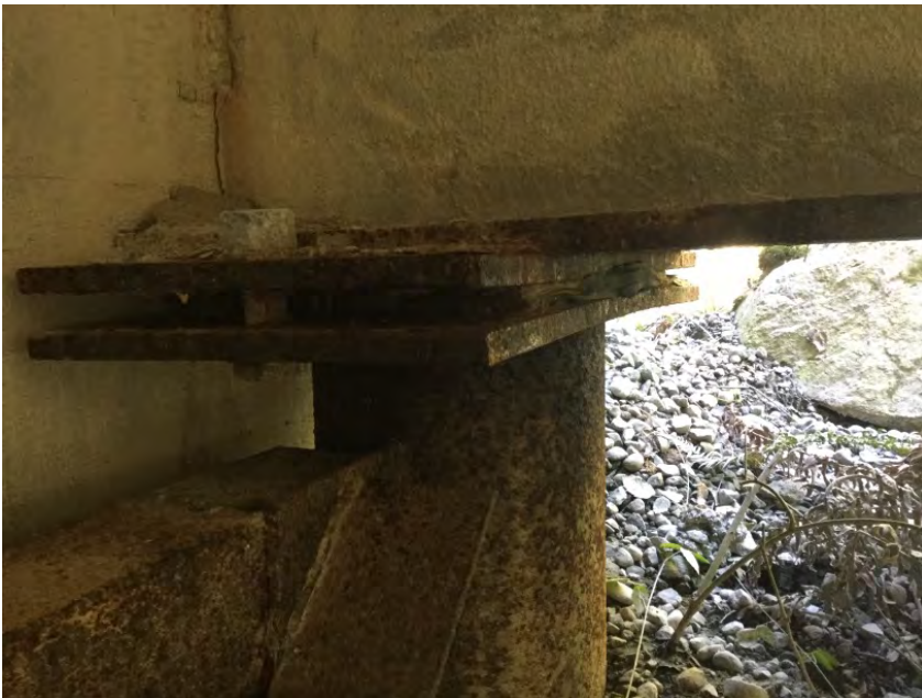
Minor bulging of bearing pads at right bank, and slight deformation noted
